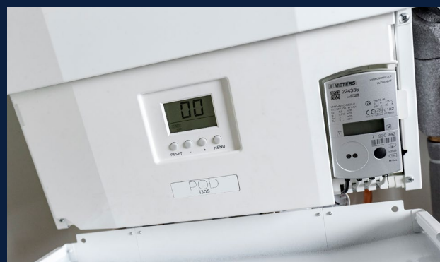
The POD HIUs have been fitted with first fix kits and factory fitted hard wired Mbus heat meters.
